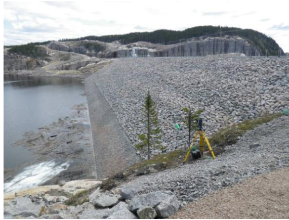
Figure 4: Side view of the Romaine-2 dam at half loading. The GNSS base station is located on the geodetic control point
